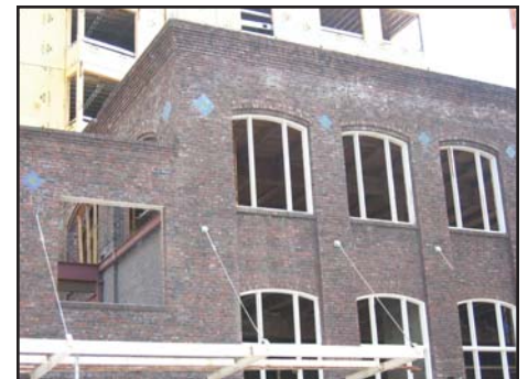
A portion of the Alley 24 project in South Lake Union is adapting the historic Richmond Laundry Building to a new use.
